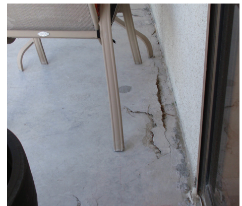
Reinforcing steel corrosion and concrete distress at balconies prior to repair
