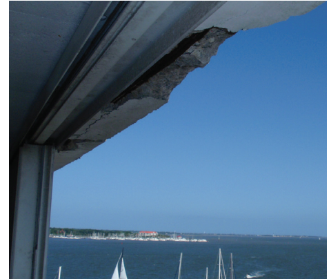
Slab edge distress and overhead spalling hazards prior to repair
