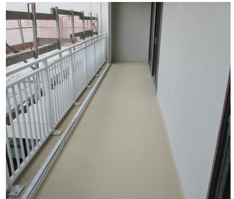
Finished balcony showing new guard rails, completed repairs and new deck coatings
