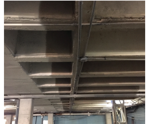
Thermal spray cathodic protection by the System Provider at garage components under the building
